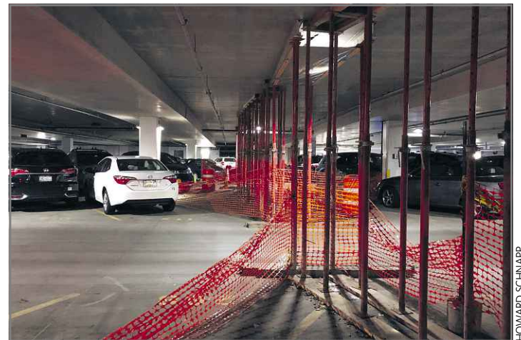
The parking garage at the Long Island Rail Road's Hicksville station, shown here in April, is open after more than three months of repairs.
